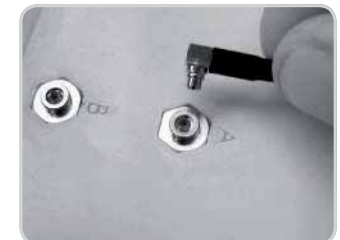
Disconnect Pigtails from the Antenna. Done :)
